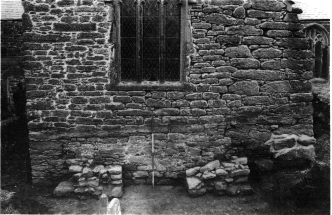
Fig 14 Lower part of the north wall of the transept, showing the foundations of the former north tower exposed during drainage works. The three main phases of construction of the wall are clearly seen: left, the original masonry and quoin; centre, infill, refacing and new window following the removal of the tower; right, rebuilt quoin and added buttress. (Photo: Warwick Rodwell)
