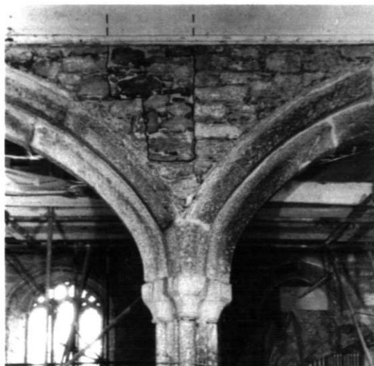
Fig 9 Detail of the north side of the nave arcade, after plaster stripping, showing the stepped infill (emphasized) of the rood-loft passage leading from the nave to the south aisle.
